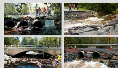
Clockwise from top left: First replacement culvert (2006); culvert failure due to Tropical Storm Ivan (2011); temporary temporary replacement culvert (2011); replacement bridge (2016).
